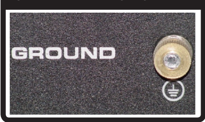
Figure #1 - Grounding Lug Block
