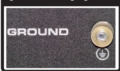
Figure #1 - Grounding Lug Block
